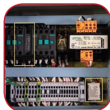
Smart electrical panel
